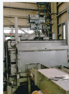
Exterior View of Equipment
