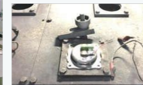
Exterior View of Equipment
